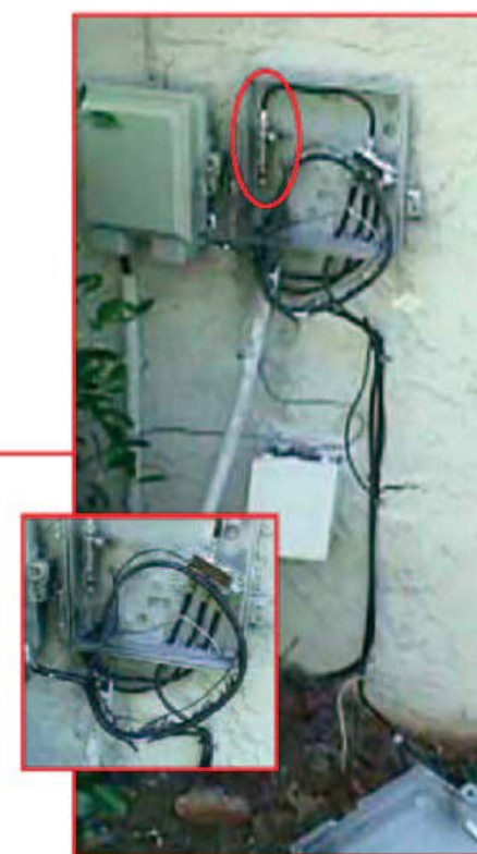
At the subscriber's home, the surge was suppressed by the TII 212 In-Line® Coaxial Surge Protector (circled). Thus, all residents in the home were safe and all equipment protected.
