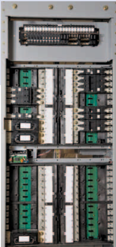
Distribution Bay with Fuses and Breakers Installed
