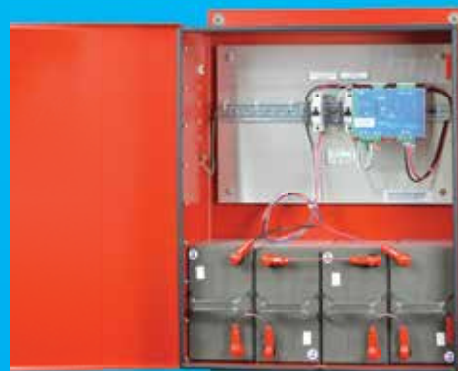
Public Safety DAS Power Enclosures
